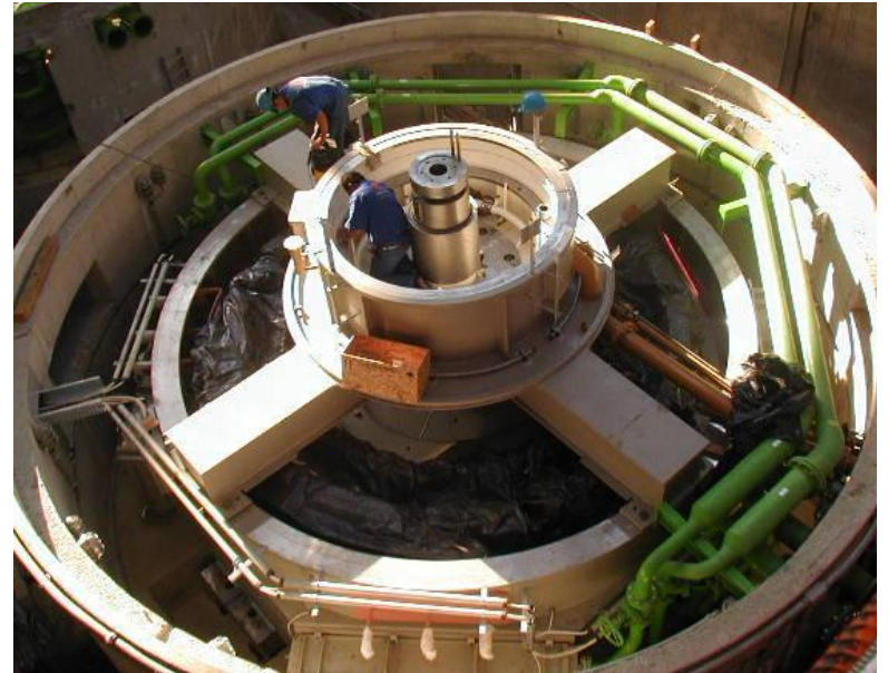
Not radially supported on concrete
